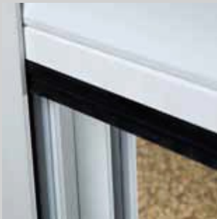
Weather seal on the bottom slat of door.
